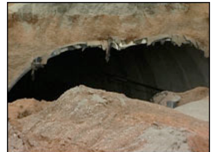
Tunnel collapse exposed residents to health threats?
